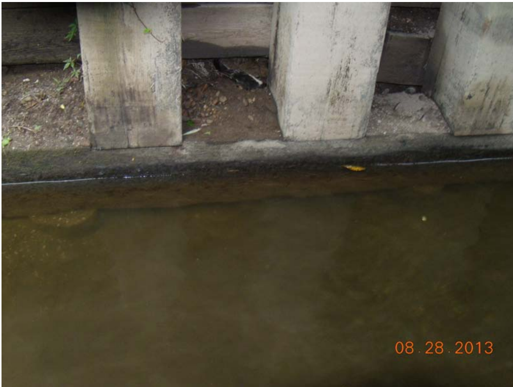
South Pier/Bent Exposed Footing & Timber Piles
