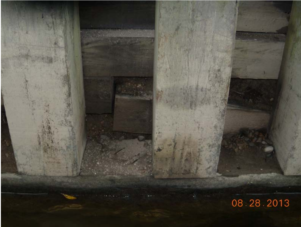
South Abutment/Retaining Wall Settlement of Timbers
