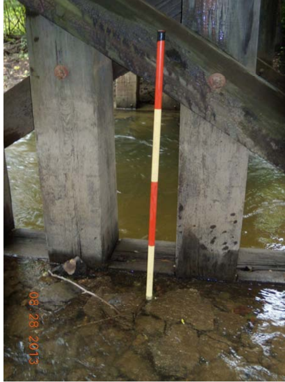
Second Pier/Bent from the South Stone / Rip Rap protection on South Side
