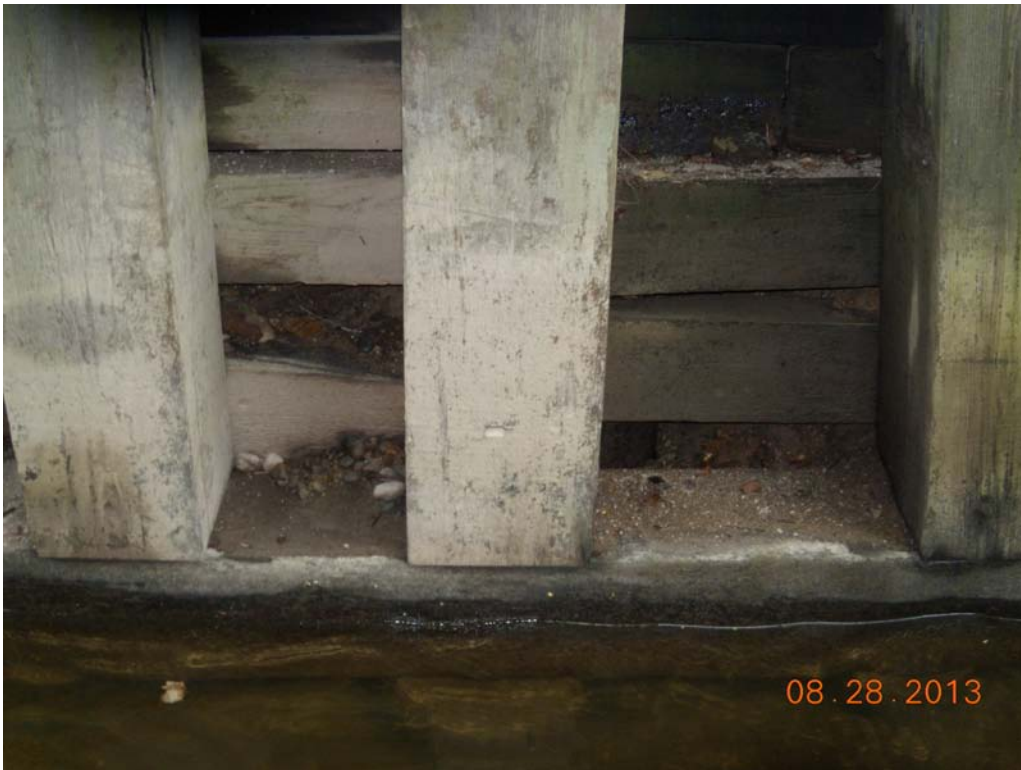
South Abutment/Retaining Wall Joint Openings / Holes
